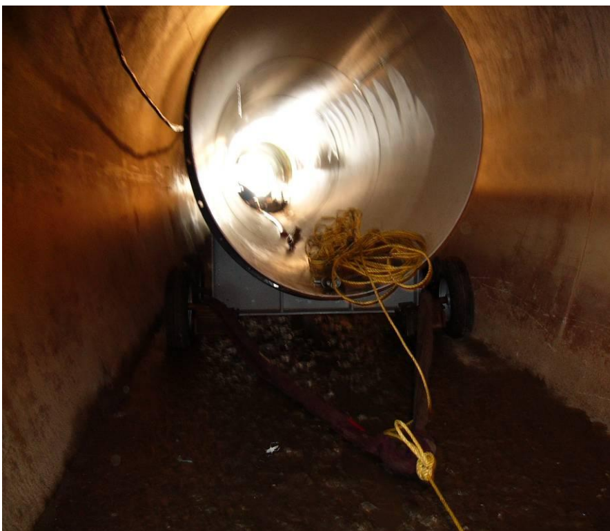
Penstock piping in the process of being winched up an existing tunnel. PFS design of temporary works.
