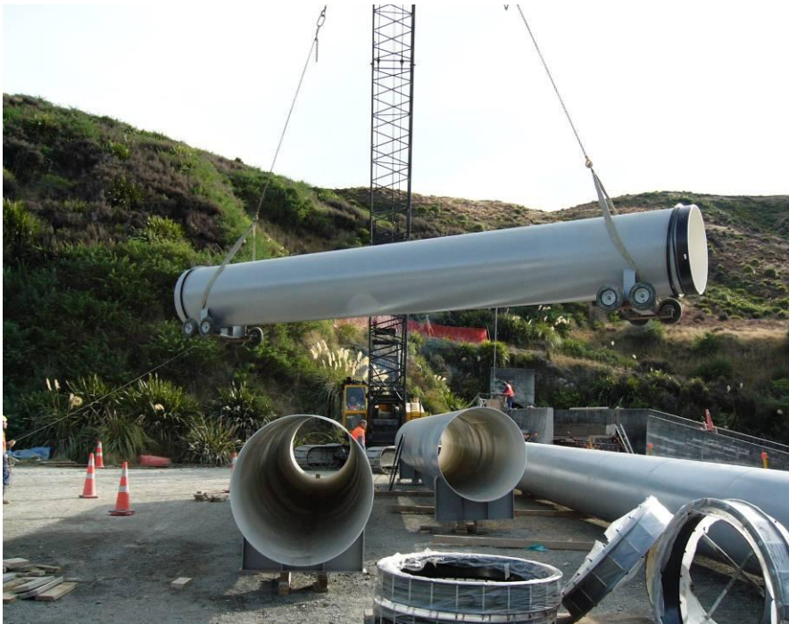
Penstock piping being lifted over the existing outfall channel ready to be pulled on the tunnel.
